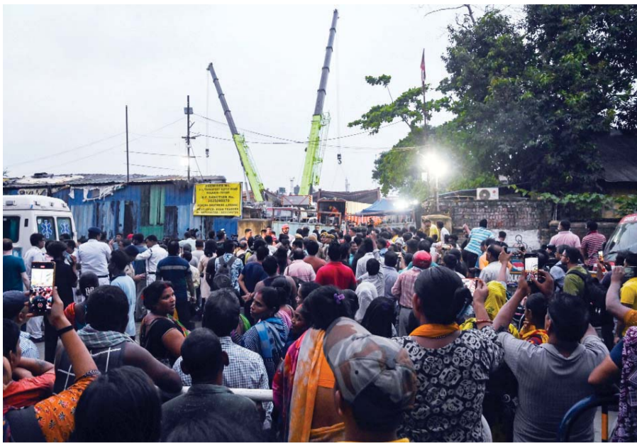
Officials with a sniffer dog conduct a rescue operation after a three-storey under-construction warehouse collapsed at Taratala area in Kolkata, West Bengal
