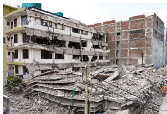
Debris of the three-storey commercial building that collapsed on Saturday evening in New Delhi
