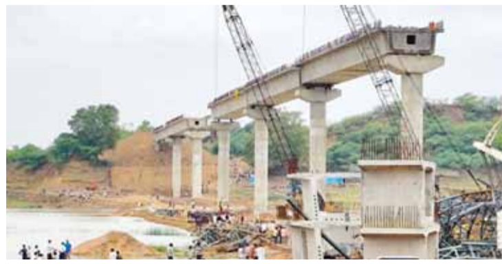
Locals gathering at the site after part of an under-construction bridge collapsed following a storm over the Betwa river in Hamirpur PTI
